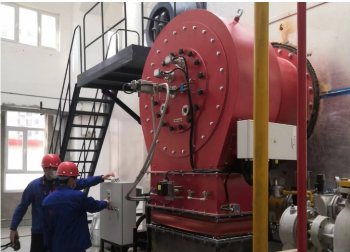
汇达热力某站40吨 Tianjin Huida-heat supply station 1 set of 40 tons
