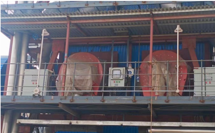
江联重工，100吨锅炉项目配套 2台60吨燃烧器 Jianglian Heavy Industry's 100 t/h boiler project is equipped with 2 sets of 60 tons
