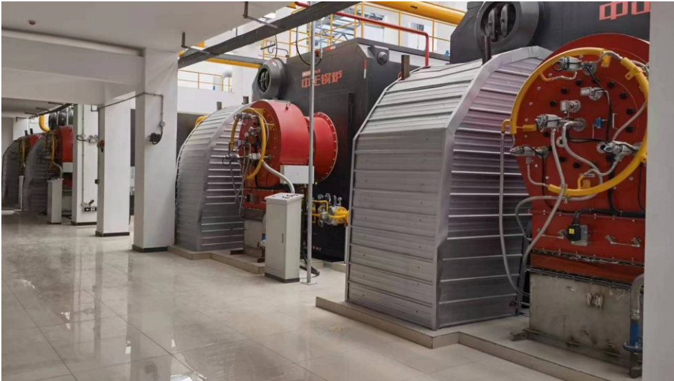
汇达热力某站4台40吨项目 Tianjin Huida- heat supply station 4 sets of 40 tons
